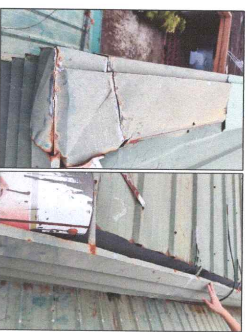
EXISTING COVERED COURT GUTTER EXHIBITS SIGNIFICANT PHYSICAL DEFORMATION, INCLUDING CRUSHING, DENTING, AND CRUMPLING, PARTICULARLY AT THE CORNER AND END CAP
