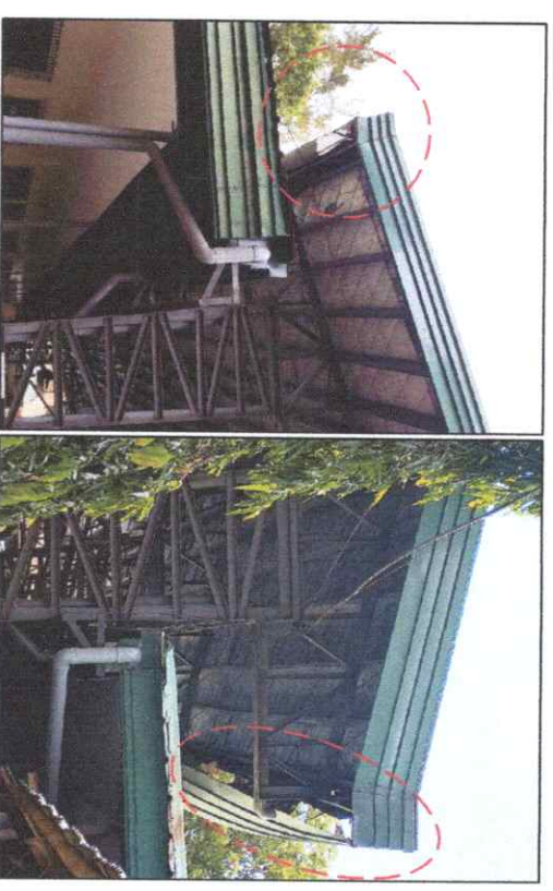
EXISTING COVERED COURT GUTTER NOTE: THE DETACHMENT IS SUBSTANTIAL, RENDERING THE GUTTER NON-FUNCTIONAL FOR WATER DIVERSION.
