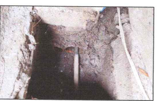
SOIL DEBRIS INSIDE CATCH BASIN NOTE: FOR DECLEGGING AND REPAIR
